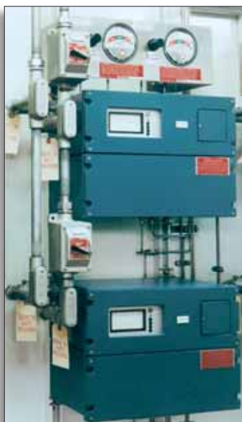
In this application, a dual pressurization system is mounted above two identical devices that are separately protected to allow independent access. Both devices feature TYPE 4 cases, which makes them suitable for purging as is.
